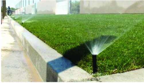
(a) Lawn irrigation sprinklers
